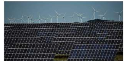
The photograph shows photovoltaic solar panels and wind turbines in the background around the Spanish Navarre town of Migaja. AP/CEA/GETTY IMAGES
